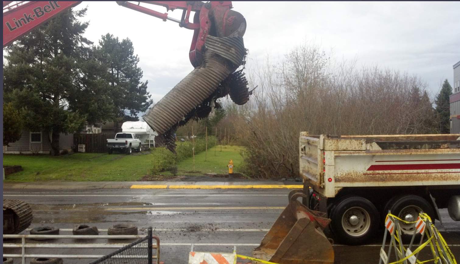
Failed Culvert @ Belmont Avenue
