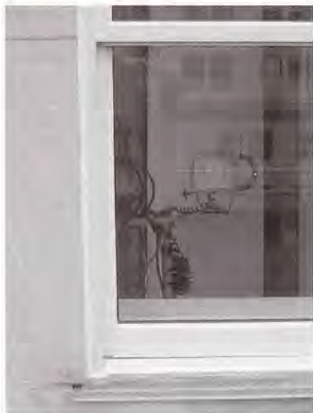
Fig. 4. Sill of the replacement window.
