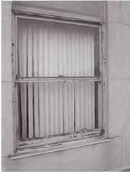
Fig. 2. View of an unrepaired steel-framed window on the east elevation of the Lafayette Building. Note the loss of paint coatings and corrosion of the built-up steel frame.
