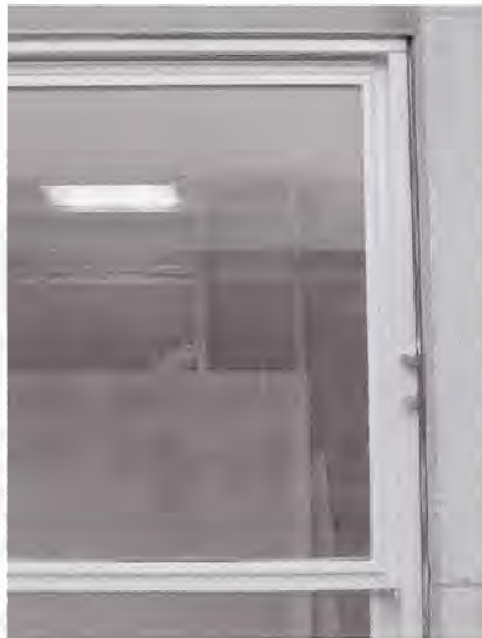
Fig. 7. Head of the repaired window. Note the similar sight lines but missing articulations and accessories of the replacement window when viewed in conjunction with the repaired window.
