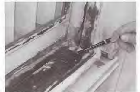
Fig. 3. View of a steel window sill on the east elevation of the eleventh floor. Note the significant corrosion of the steel frame at the sill-to-jamb corner.
