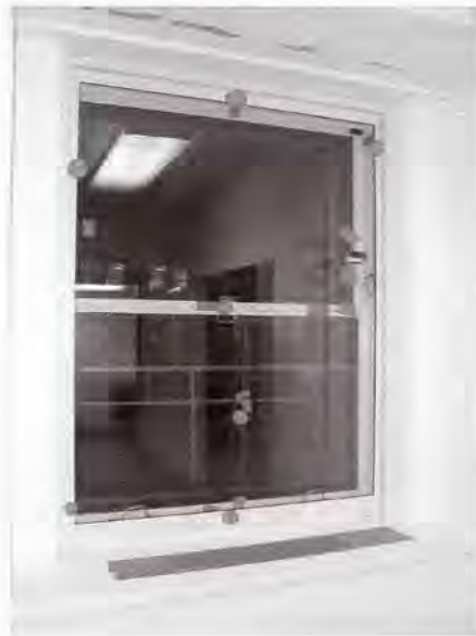
Fig. 8. Interior view of the repaired window prior to installation of the interior chamber. Note the thermal and relative-humidity sensors are indicated with dots. Some sensors are installed on the repaired window, and others are installed on the storm sash, resulting in more sensor locations than on the replacement window.
