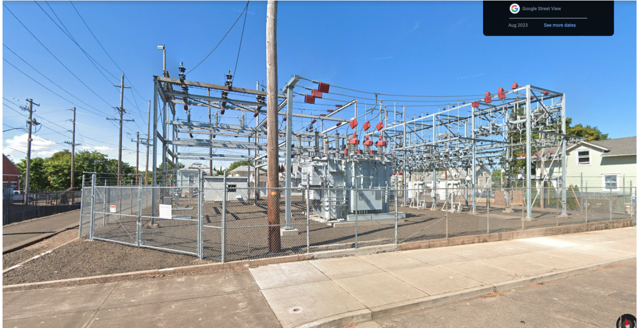
Unattractive substation - corner of 4th and Vine (Directly across from site)
